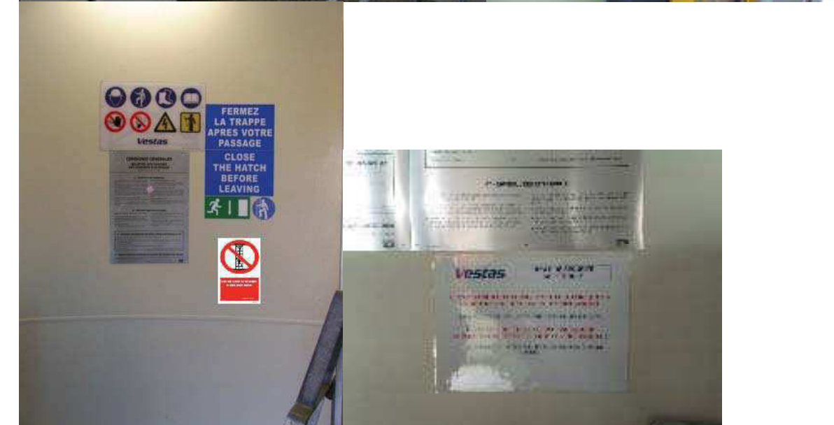
Figure 2.1.1: “Vestas Safety Panel” (item 60093470), “Electrical Safety Advice & Equipment”, “Fermez la trappe après votre passage / Close the hatch before leaving”, “Safety Harness required when climbing” (item 208056), “Emergency exit arrow down” (item 208015), “Only one person on the ladder in each tower section” (item 208058) and his translation, “Consignes de sécurité électriques” “Safety rule Ladder/Service lift” Place the signs to the left of the ladder.
