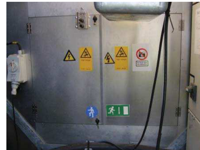
Figure 3.1.2: “Emergency Exit Arrow down” (item 208015), “Safety harness required” (item 208006) Place the signs on the partition wall to the transformer room “High Voltage” (item 208057) and his translation, “No flash photographing” (item 208009), “Electrical Hazard” (item 208013) Place the signs in the centre of the hatch to the transformer room
