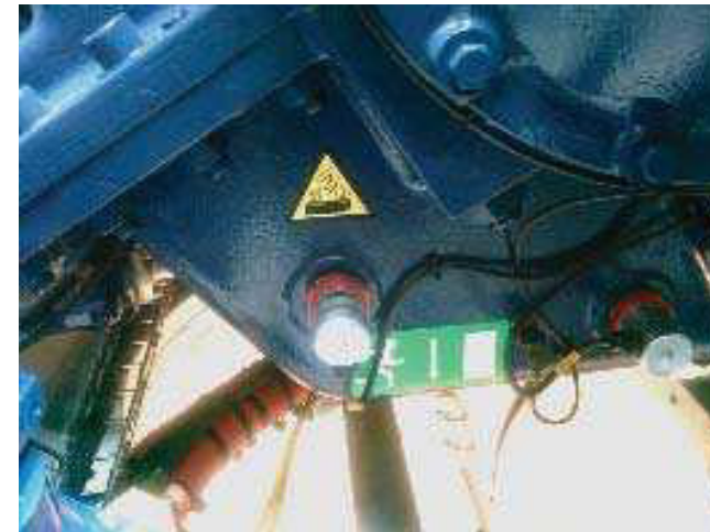
Figure 3.3.4: “Hot Surface” (item 208023), “Emergency Exit Arrow Down” (item 208015) Place the both signs on the lower part of the back of the gearbox (above the ladder going down to the top platform).
