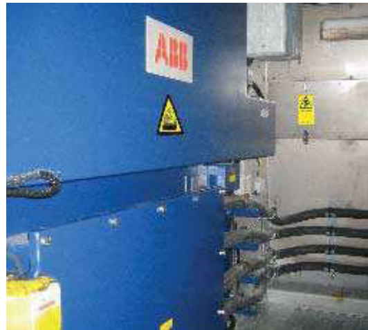
Figure 3.3.5: “Hot surface” (item 208023) Place the sign on the middle of the air-to-air cooler on the generator
