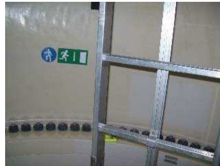
Figure 2.2.1: “Emergency Exit Arrow down” (item 208015), “Safety harness required when climbing” (item 208056) Place the signs on the left side of the ladder, approximately 170 cm above the platform
