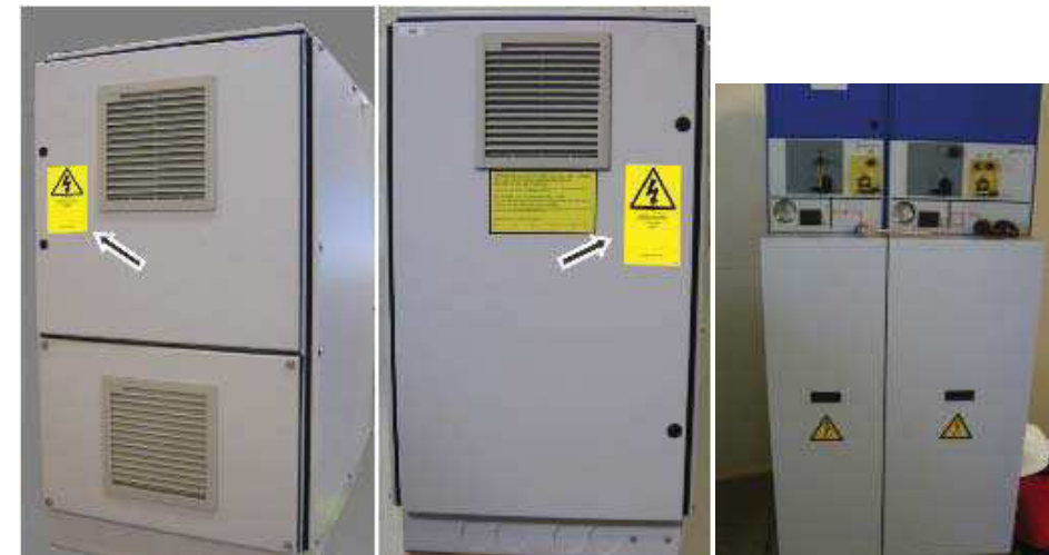
Figure 2.1.5: “Caution ! Battery voltage remains on after deenergizing” (item 119078) and his translation Place the signs on the UPS system - “Electrical Hazard” (item 208013) Place the signs on the switchgear
