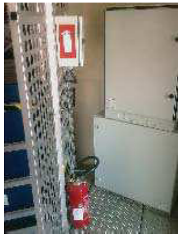
Figure 2.1.7: “Fire Extinguisher” (item 208007) Place the signs next to the lift at the bottom platform approximately 170 cm above the bottom platform
