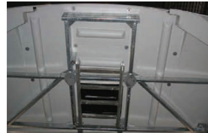
Fig. 91 Hatch and ladder in the nacelle
