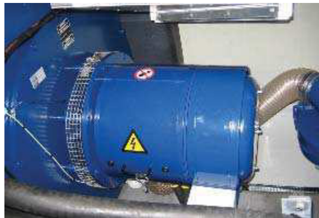
Figure 3.3.2: “Do not step here” (item 208029) on the top of the slip ring unit “Electrical hazard” (item 208013) on each cover for the slip ring housing
