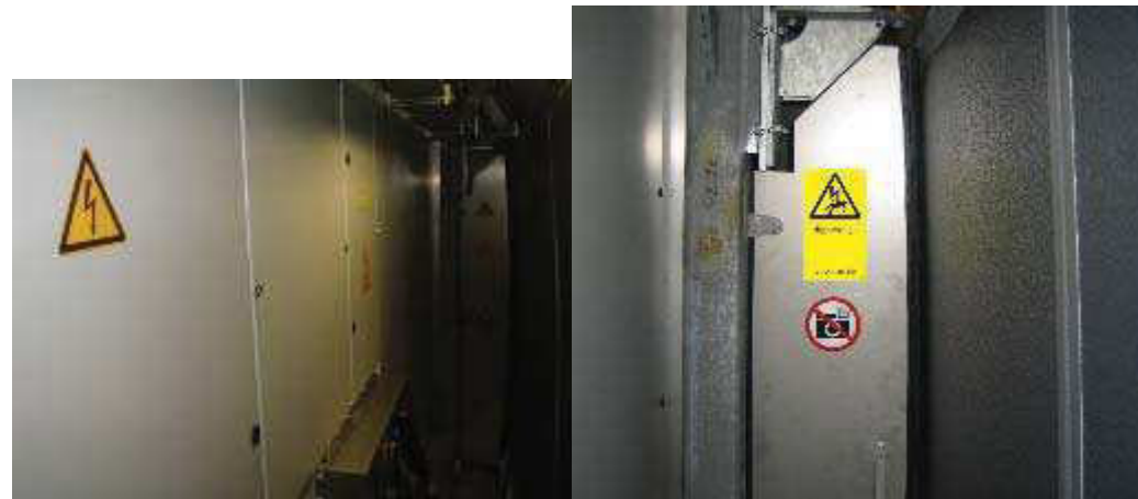
Figure 3.2.5: “High Voltage” (item 208057) and his translation, “No flash photographing” (item 208009) Place the signs on the door to the transformer behind the controller cabinets “Electrical Hazard” (item 208013) behind the controller cabinets
