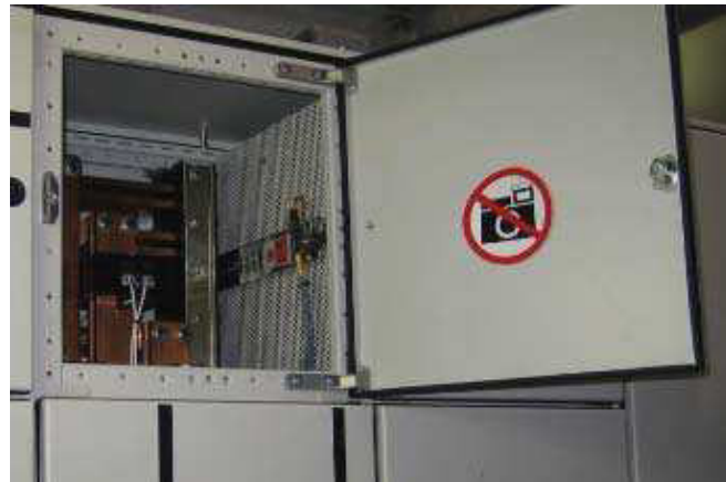
Figure 3.2.4 “No flash photographing” (item 208009) Place the signs on the inside of the cabinet door above the Q8 breaker.
