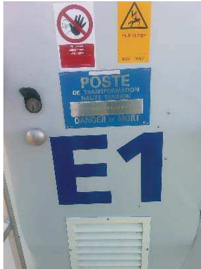
Figure 1.1: “No Access for Unauthorized Personnel” (item 208003) and his translation, “High Voltage” (item 208057) and his translation, “WTG Number”, “Poste de transformation” Place the signs on the door
