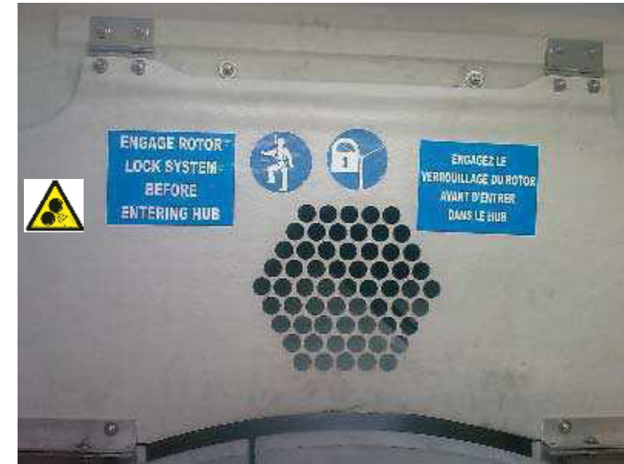
Figure 3.4.1: “Rotor Lock Required” (item 208027), “Rotating Parts Behind” (item 208017), “Safety Harness required” (item 208006), “Engage rotor lock system ... / Engagez le verrouillage du rotor” Place the signs on the partition wall to the hub. Place the signs to the left just above the hatch.
