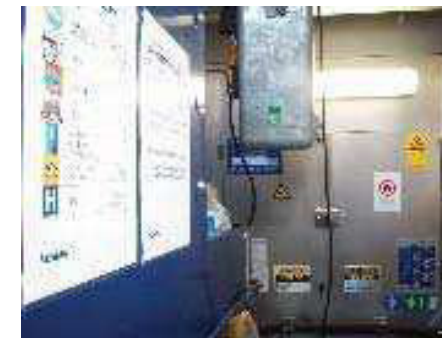
Figure 3.1.1: “Emergency Plan” Place the sign on the generator.
