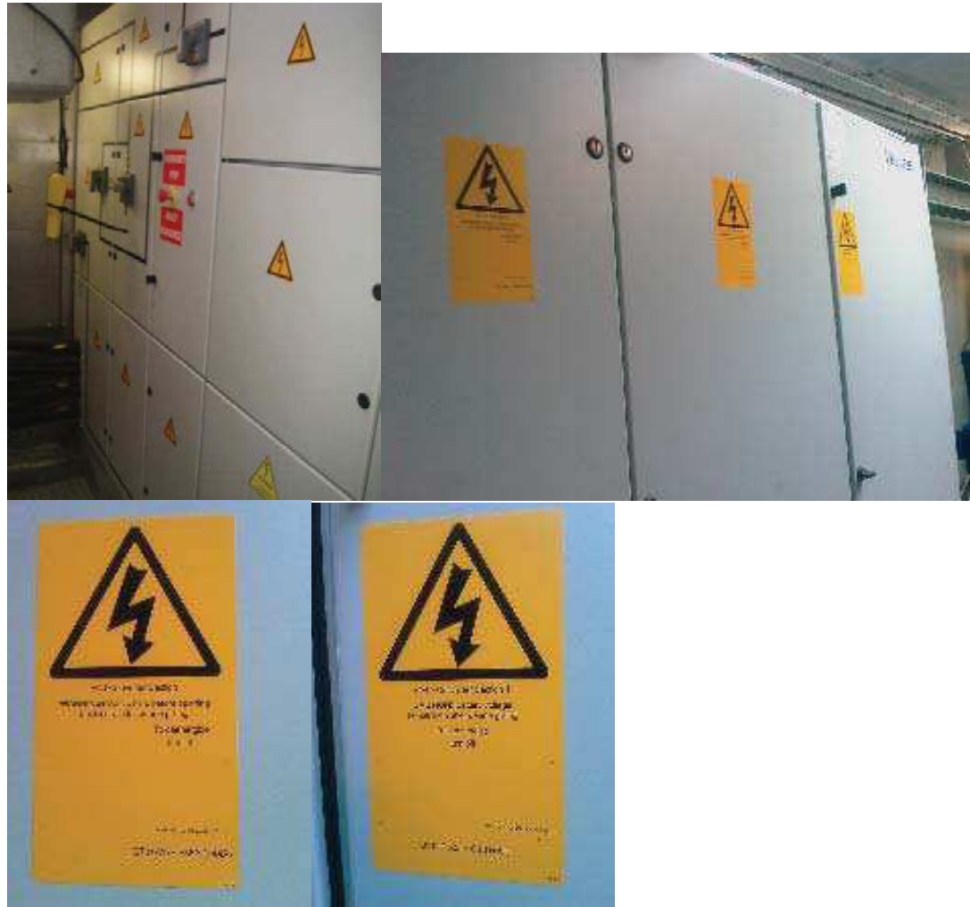
Figure 3.2.1: “Electrical hazard” (item 208013), Warning wait 5 min ...” (item 119079) and his translation, “Caution Battery voltage ...” (item 119095) and his translation Place the signs on the top controller.
