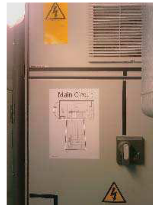
Figure 3.2.3 “Main circuit” (item 119081) Place the signs on the top controller near the Q16 breaker
